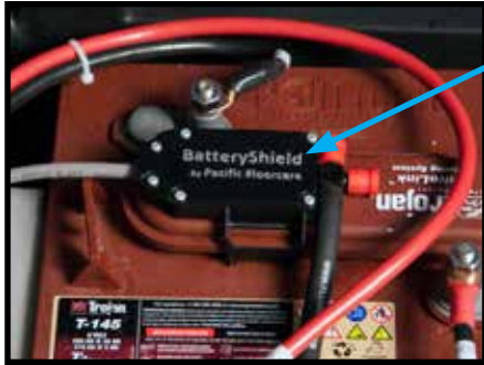
BatteryShield optical sensor on Trojan battery
